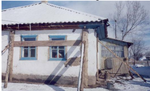
Photo 5 : DAMAGES OF THE HOUSE IN SUMBE VILLAGE (□ degree area, house destruction)
