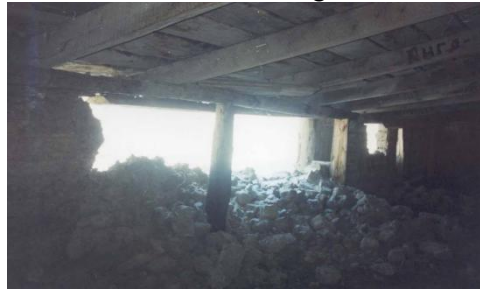
Photo 6 : COLLAPSE OF THE SHEEP-FOLD WALL IN SUMBE VILLAGE (□ degree area, Sheepfoldwall collapsed)
