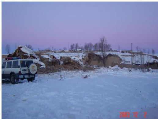
Photo 3: The collapse of the civil structure
