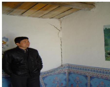
Photo 8: Cracks in the corner of the houses of the 1st village of Hetuhaoer Township, in the VII degree
