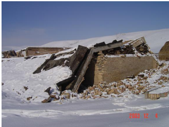
Photo 11: Entire collapse of sheep pen No. 1 in VIII degree
