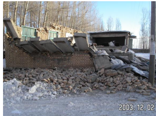
Photo 10: The School of the 1st village of Hetuhaoer Township in District VIII collapsed
