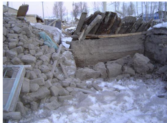
Photo 4: The collapse of the civil structure
