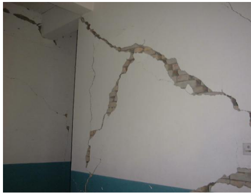
Photo 9: "X" crack in the cross wall of the HuiWu station office building in the VIII degree area
