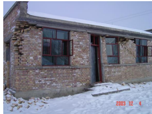
Photo 12: Reversed damage of newly built houses in VIII degree area
