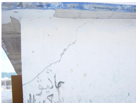
Photo 7: Cracks in the corner of the house of Aksu village in the VII degree district
